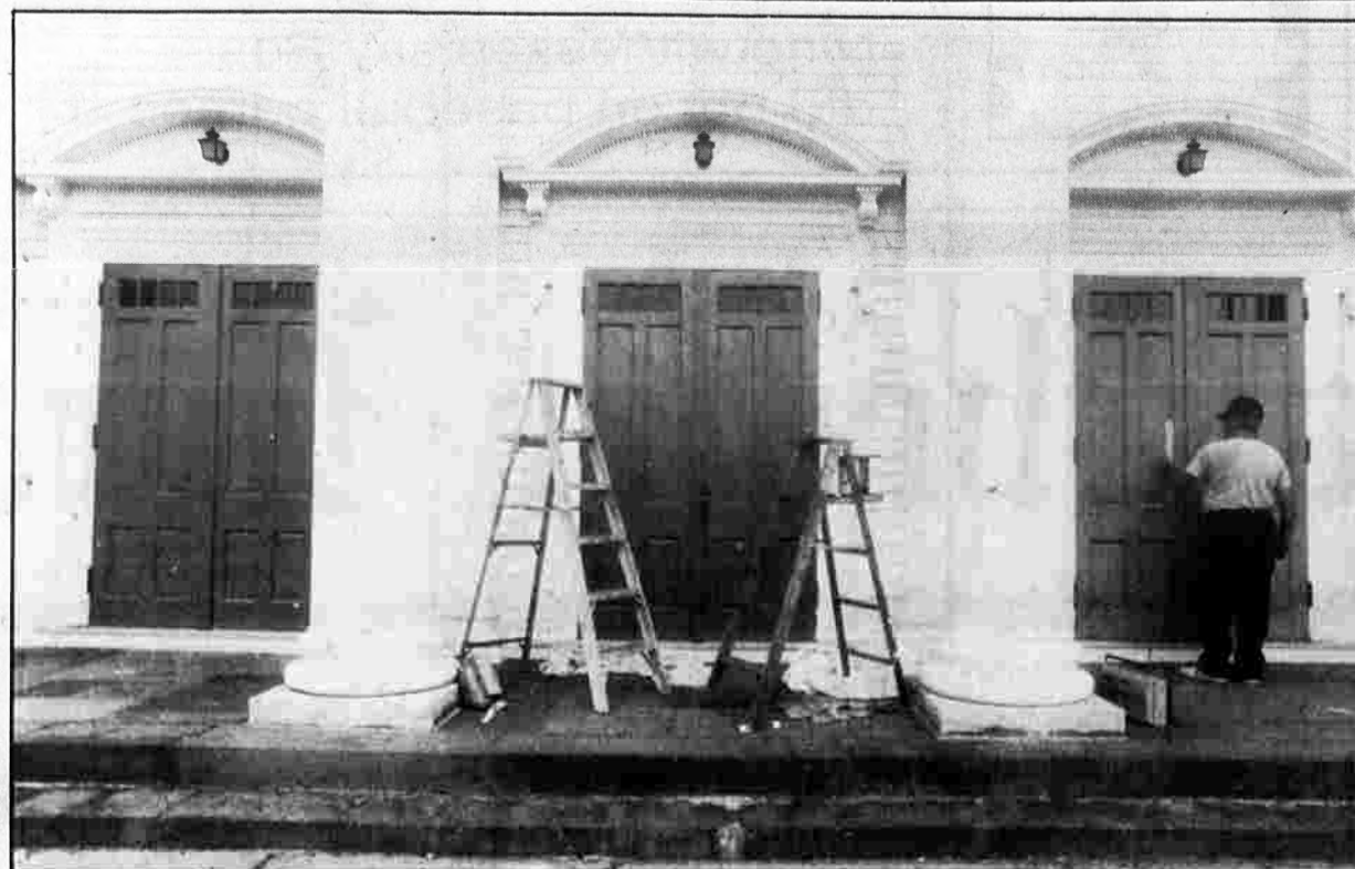
REPAIRMAN — Ken Pelletier of 41 Case Drive caulk a door Wednesday at Center Congregational Church, 11 Center St.
